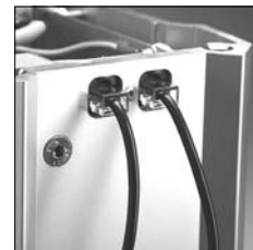
Anschluss der Synchro-Kabel in der Reihenschaltung einer Gruppe. Connecting the synchro cables between the members of an array.
